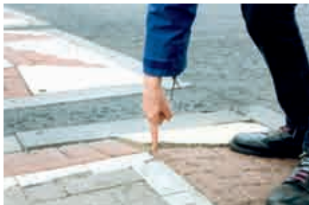
Fig. 2.8 Damage to a speed cushion
